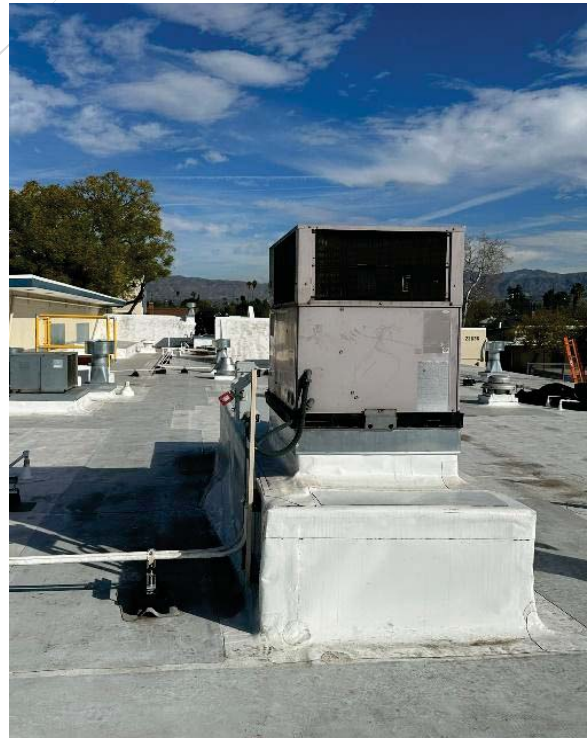
Cafeteria – CO T-503 – Swamp Cooler
